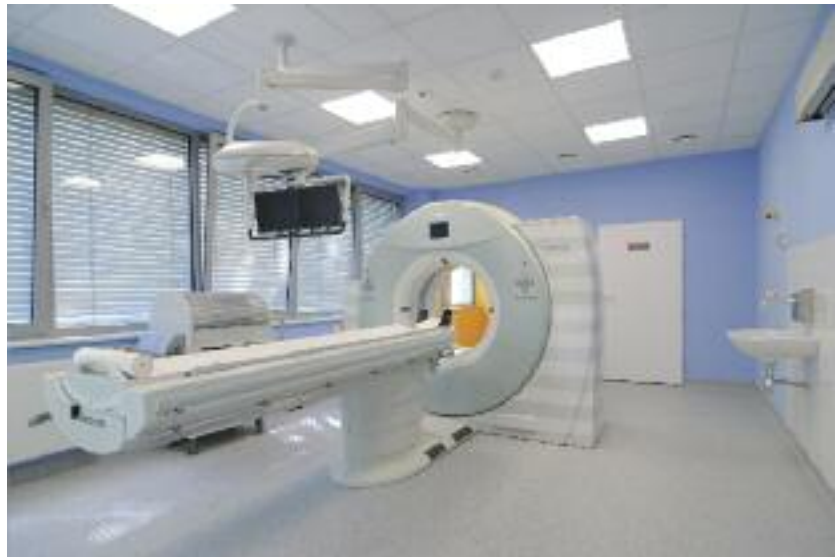
Hospital Ruzomberok (SK) - Clean Room Grid.
